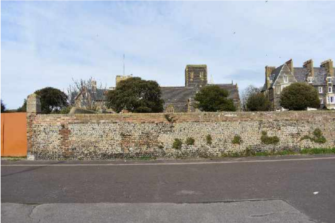
Decaying boundary walls on West Cliff promenade
