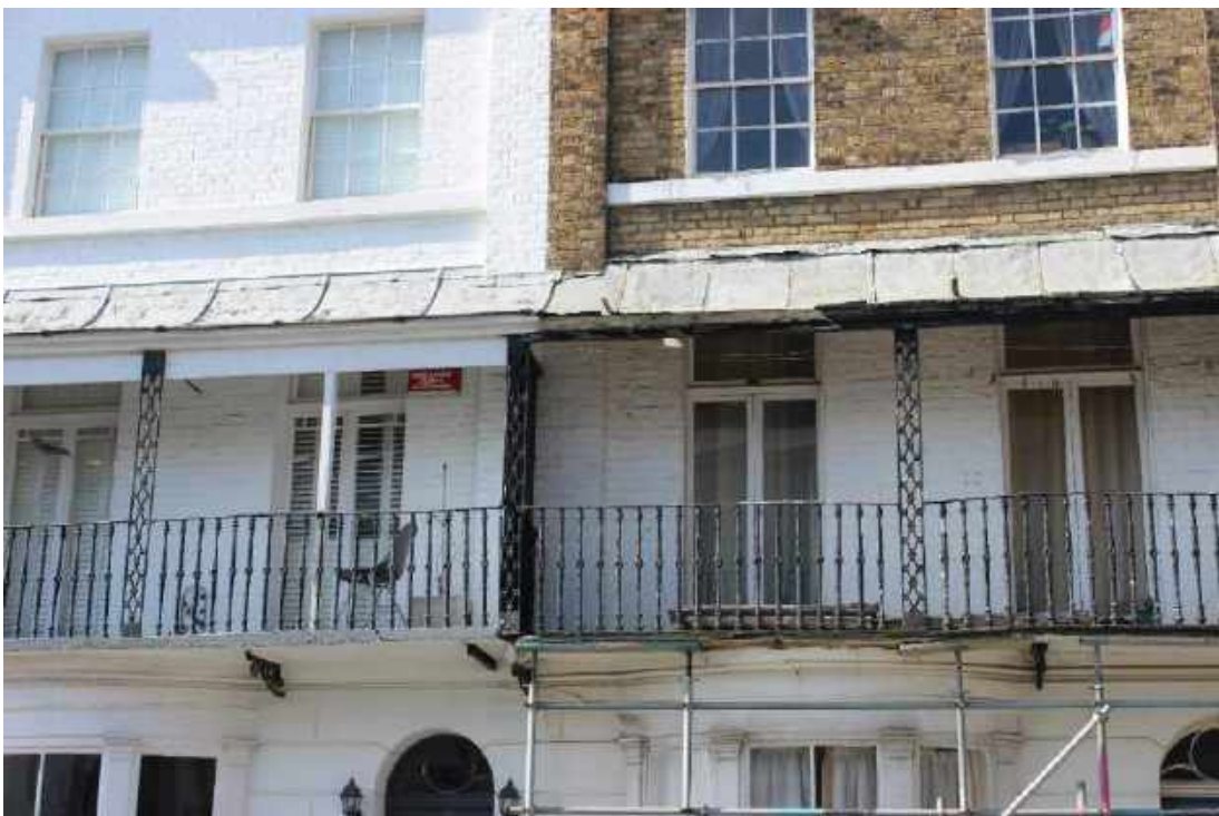
Poorly-maintained historic fabric on houses around Spencer Square
