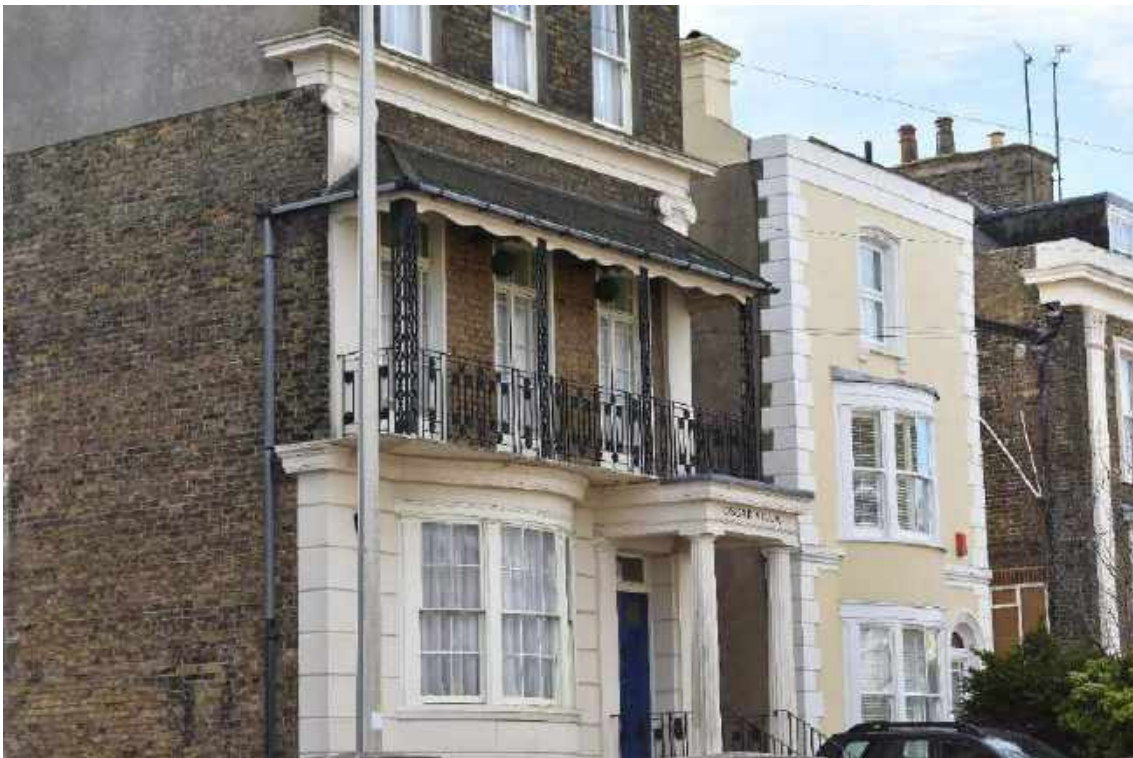
Fine-grained architectural detailing on the villas at the western end of West Cliff Road
