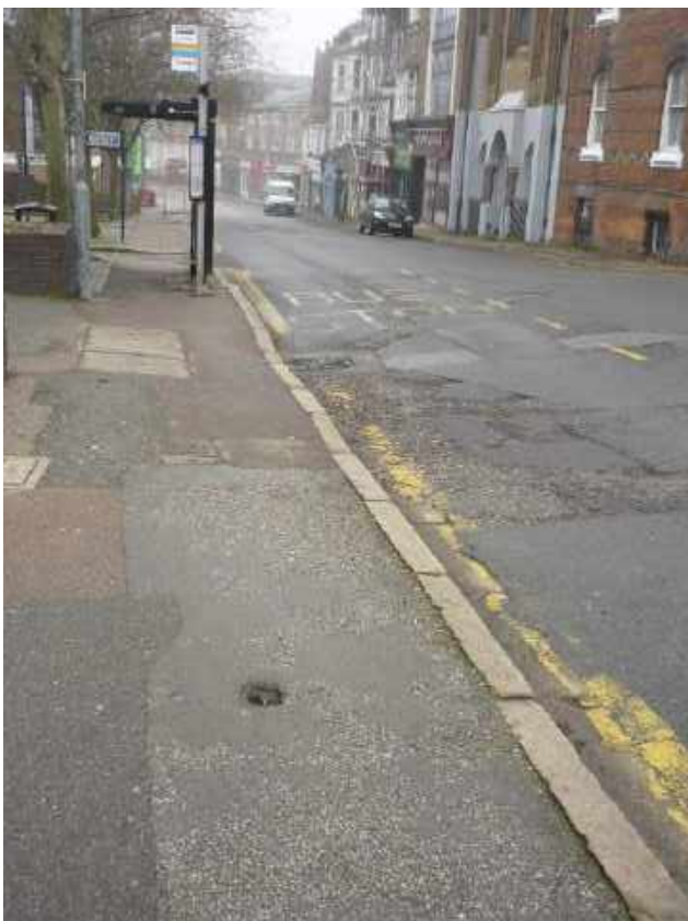
Poor quality surfaces
