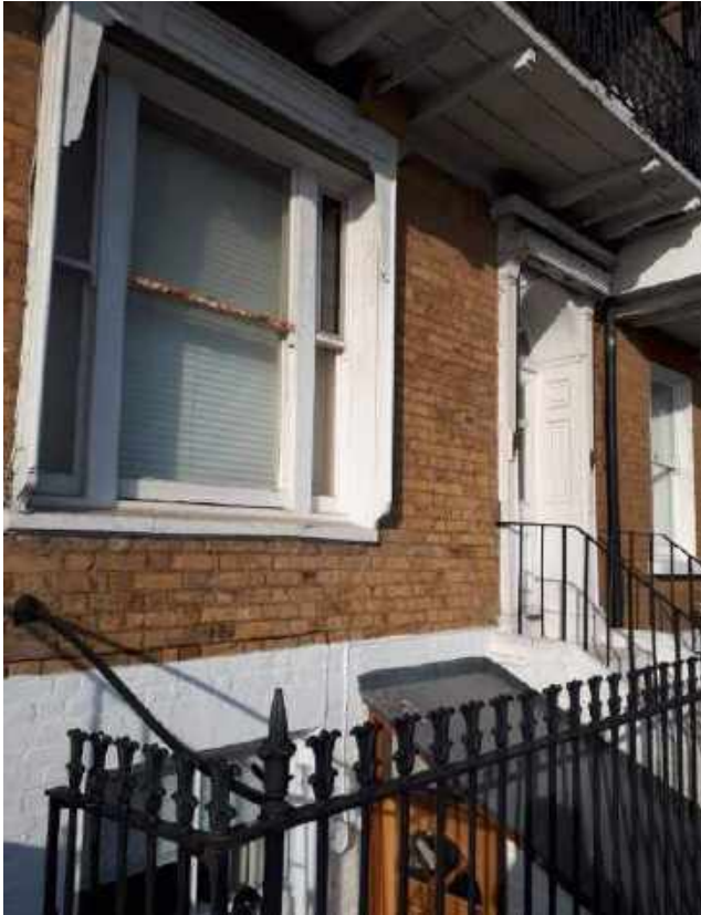
The now fixed blind boxes on this southerly facing elevation invite the reinstatement of solar shading.
