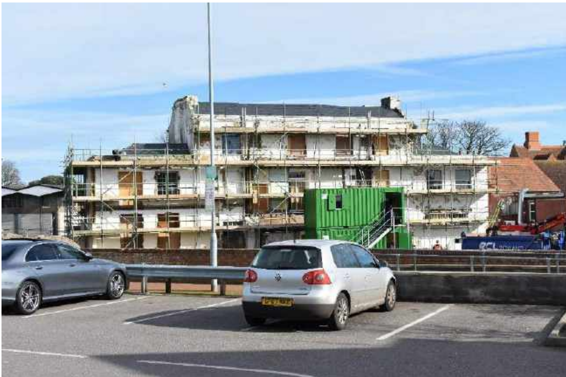
Townley House is currently undergoing a refurbishment as part of a new housing development
